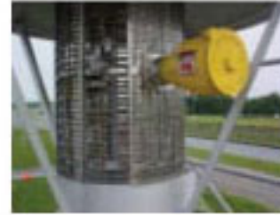
Out-freezing device on exhaust stack, ATEX classified site 1 kW
